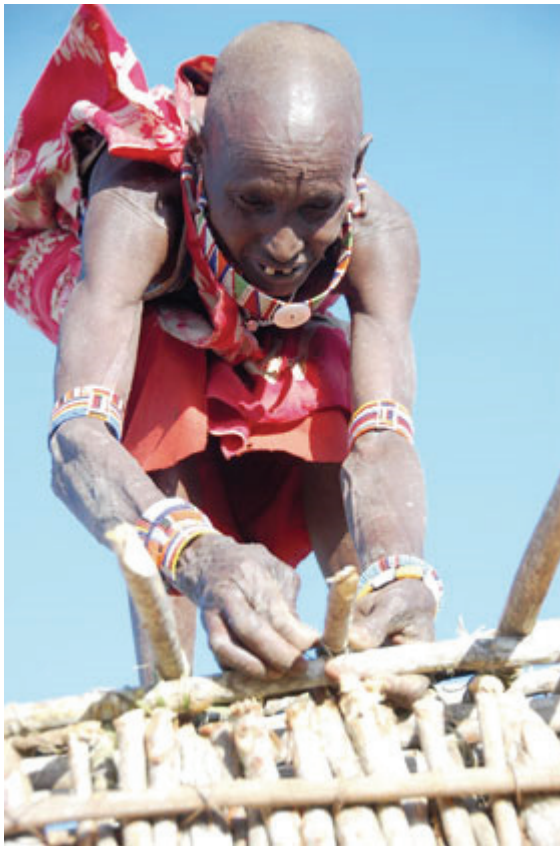
Yangaso Parmat, a Maasai woman, builds a manyatta for her son in Kajiado. It is customary for women to construct huts.
